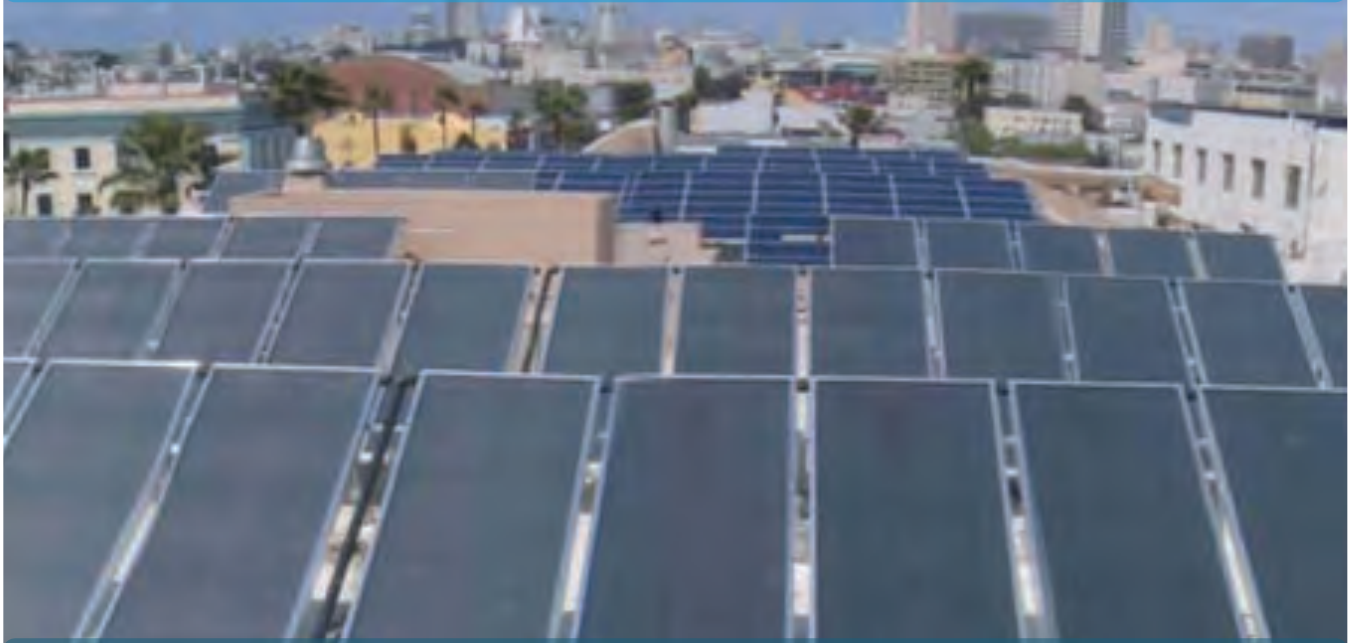
Rooftop solar thermal collectors in foreground, solar PV panels in background.
