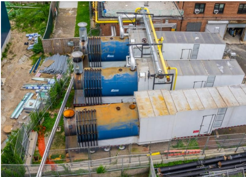
Image of critical building systems.
