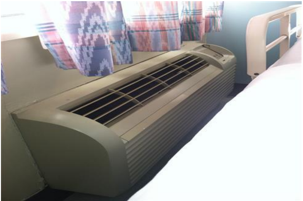
21 - RESIDENT ROOM ELECTRIC HVAC UNIT
