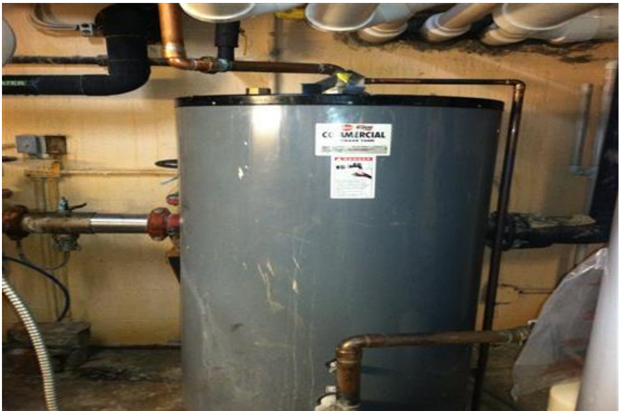
16 - DOMESTIC HOT WATER HOLDING TANK
