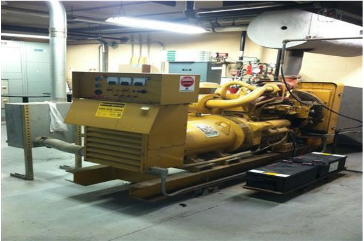
33 - EMERGENCY BACK-UP ELECTRICAL GENERATOR
