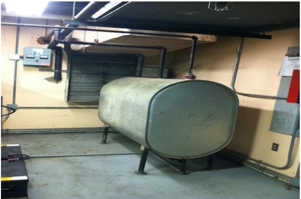
34 - DISESEL FUEL STORAGE TANK
