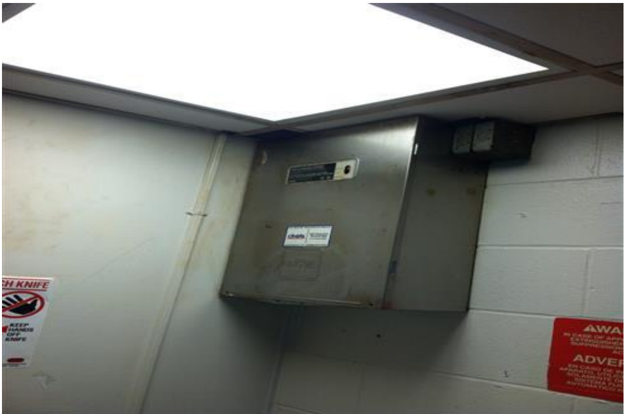
22 - KITCHEN FIRE SUPPRESSANT SYSTEM
