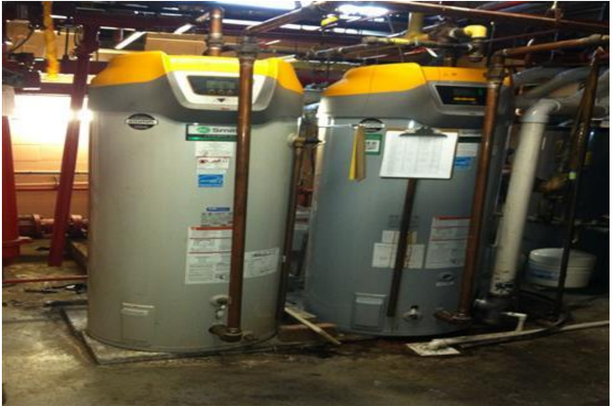
15 - NATURAL GAS BOILERS FOR DOMESTIC HOT WATER
