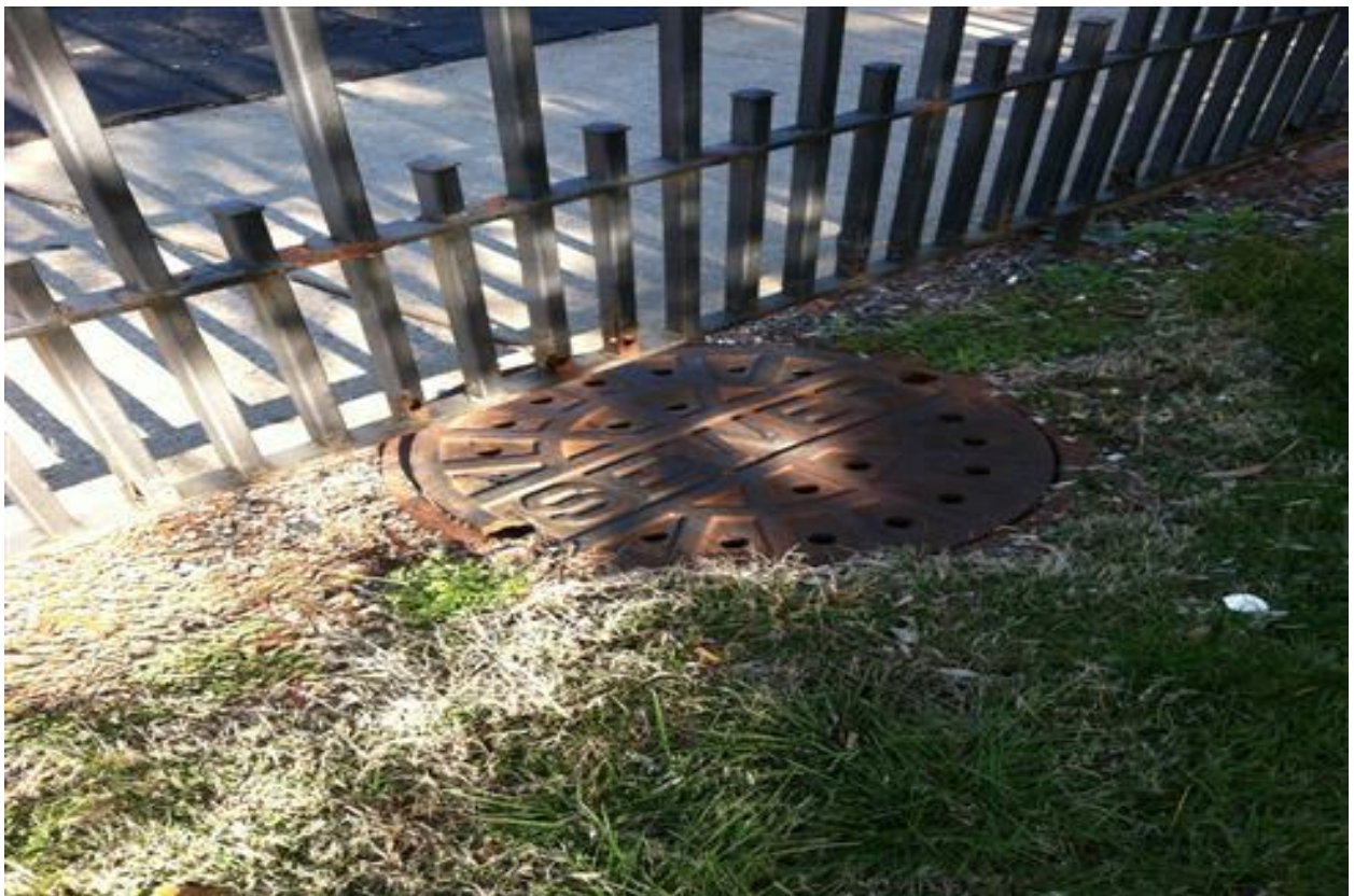
44 - PUBLIC SEWER SYSTEM ON-SITE
