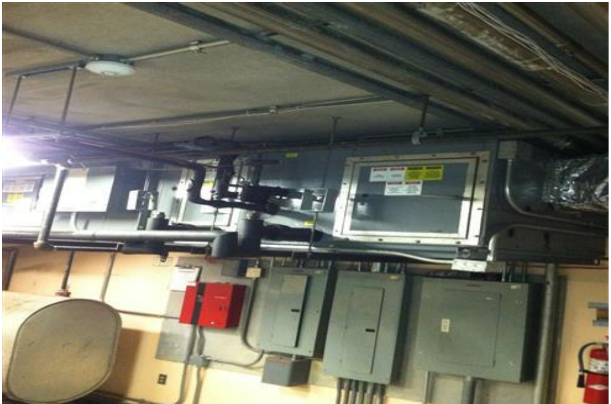
18 - SUSPENDED HVAC UNIT FOR THE BASEMENT
