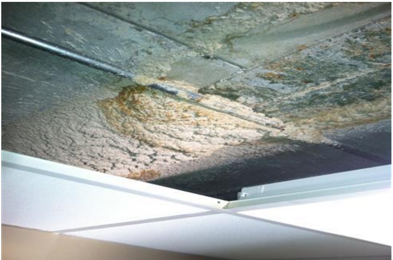
12 - SPRAY-ON FIREPROOFING ON STEEL BEAM ABOVE SUSPENDED CEILING, 3RD FLOOR
