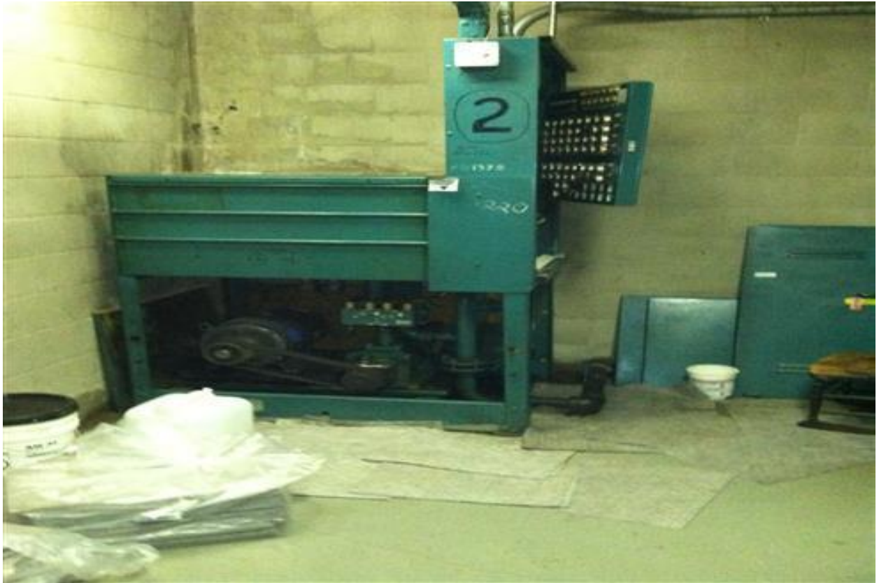
07 - ELEVATOR EQUIPMENT ROOM - ABSORBANTS USED FOR MINOR HYDRAULIC LEAK
