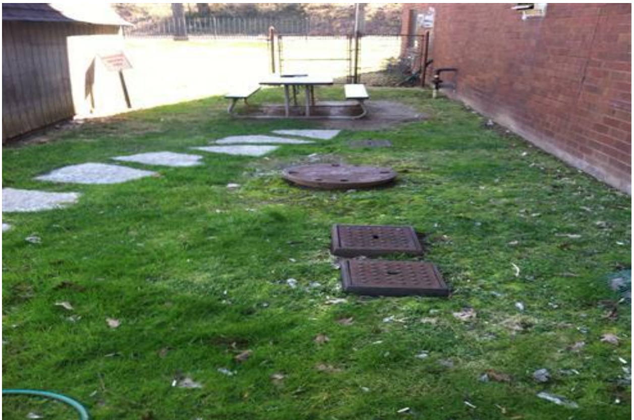
42 - UNDERGROUND GREASE INTERCEPTOR
