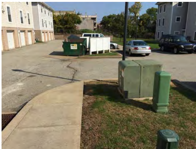
View of pad-mounted transformer and dumpster on northern portion of site
