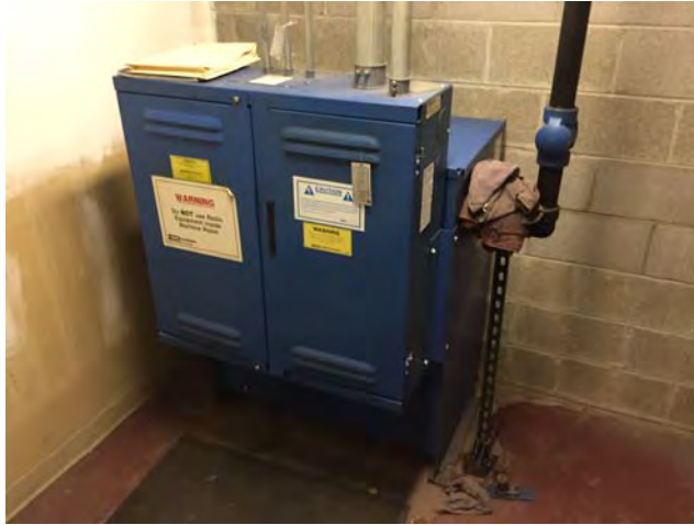
View of elevator lift system in main apartment building
