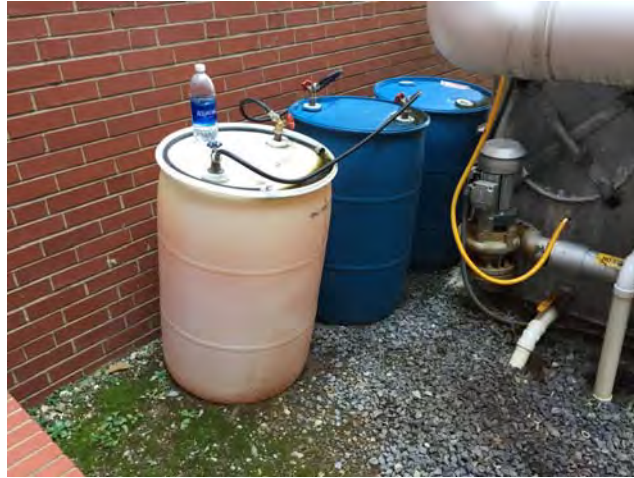
View of glycol drums staged outside adjacent to cooling tower
