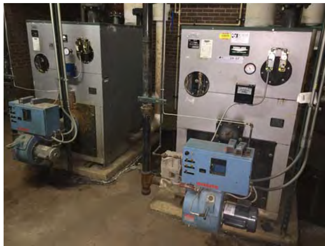
View of boilers in utility room of main apartment building
