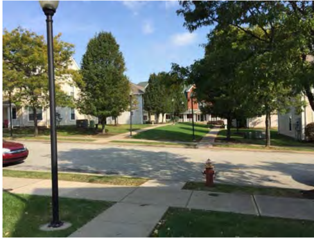
View of pad-mounted transformers and townhomes
