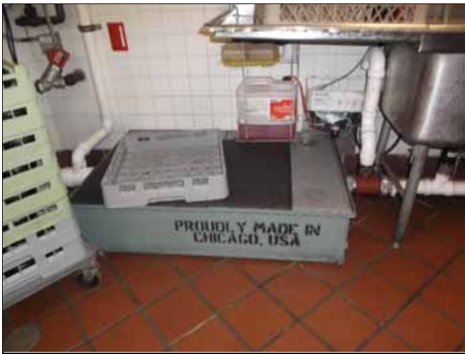
13. View of grease trap
