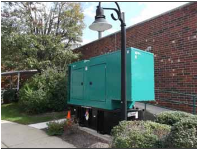
19. View of Emergency Generator
