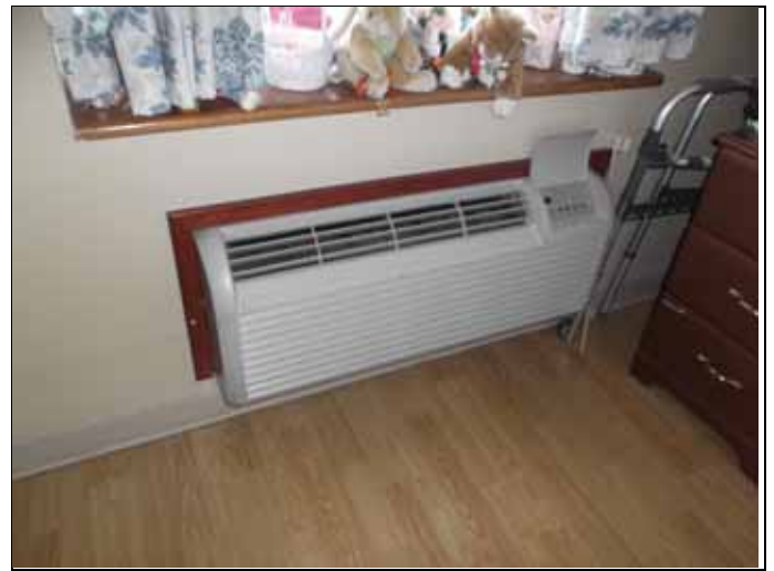
8. View of PTAC Unit
