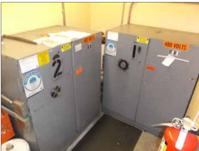
17. View of Elevator Equipment
