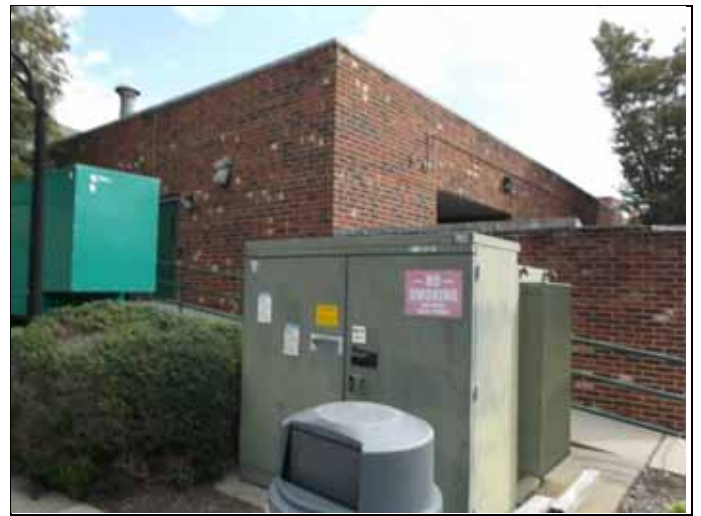
20. View of Pad-mounted Transformer
