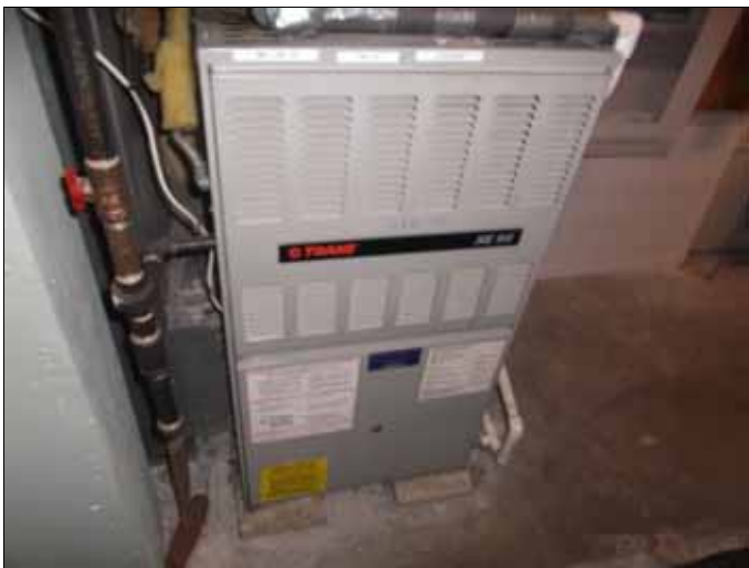
9. View Heat Pump Unit
