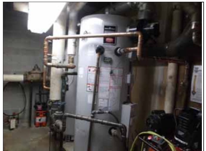
10. View of Gas Water Heaters
