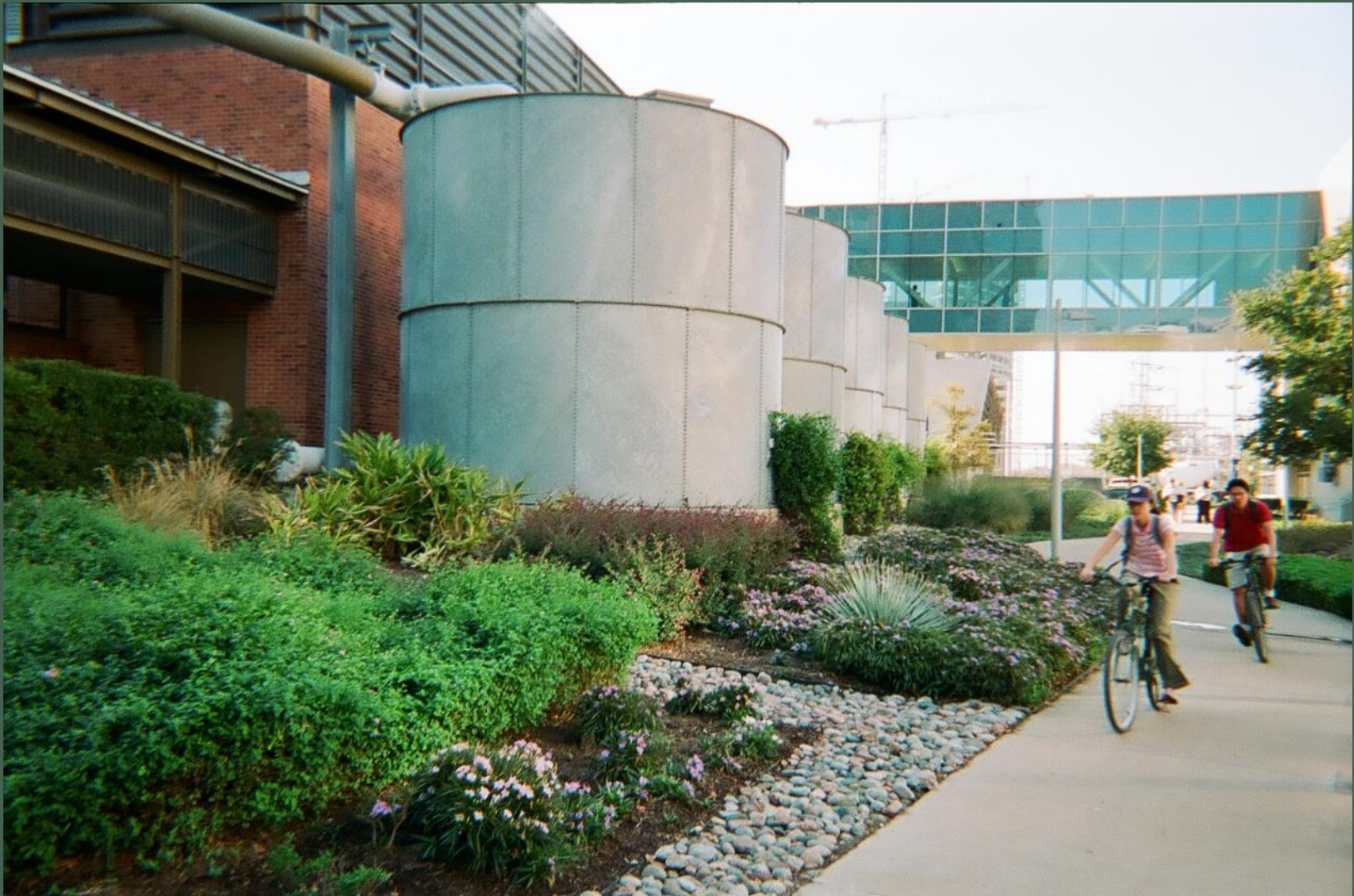
Rainwater cisterns used to capture rainwater at the Texas Medical Center School of Nursing. Photo courtesy of Suzanna Perea.
